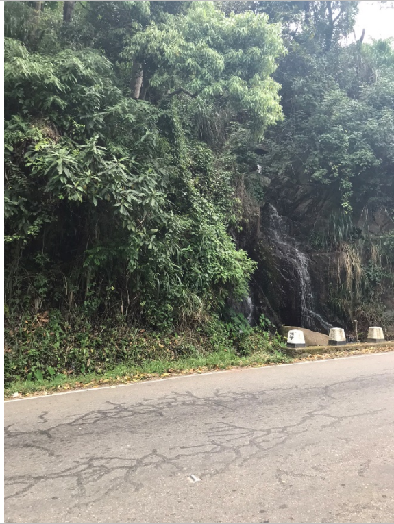
Road subsidence in the site (infront of the cutting failure)
