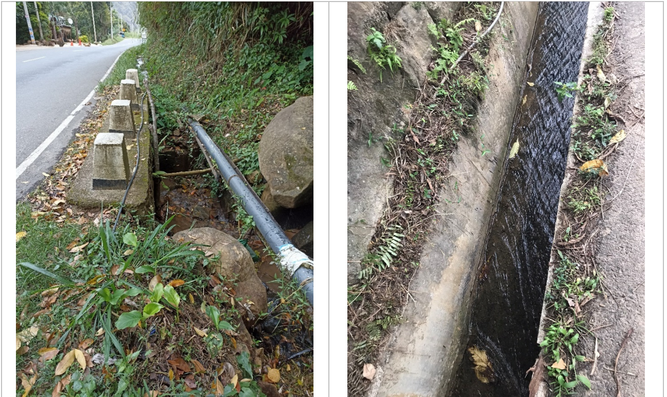
Figure 6f: Drainage and the Water supply line going through the down slope of the area
